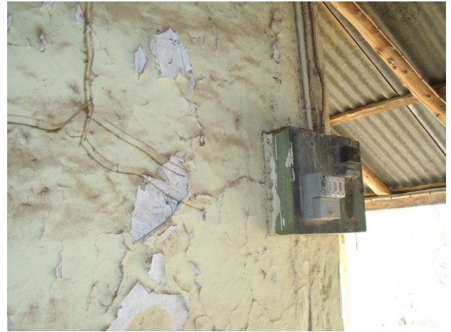
Figure 3.4. Asbestos containing electrical backboard
